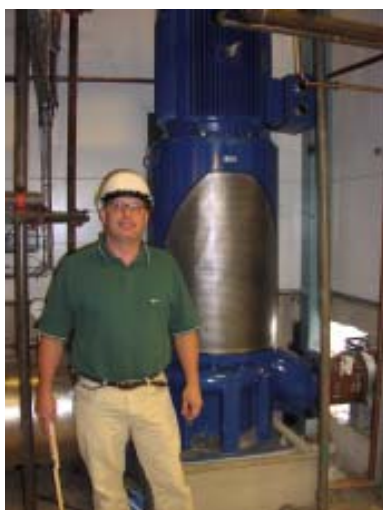
Distribution - Kungälv Energi SNLV-H 250/400
