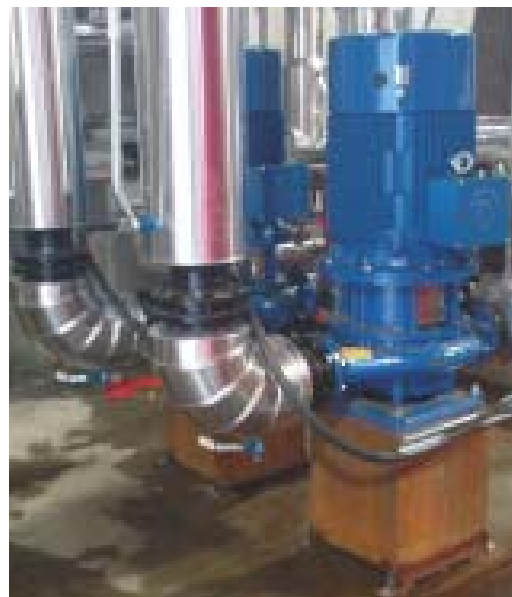
SNL, booster pump
