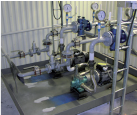
Fuel burner pump
